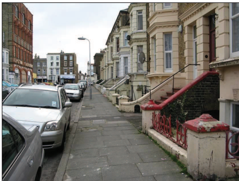
Improvements are needed to the pavements and street lights in the Conservation Area
